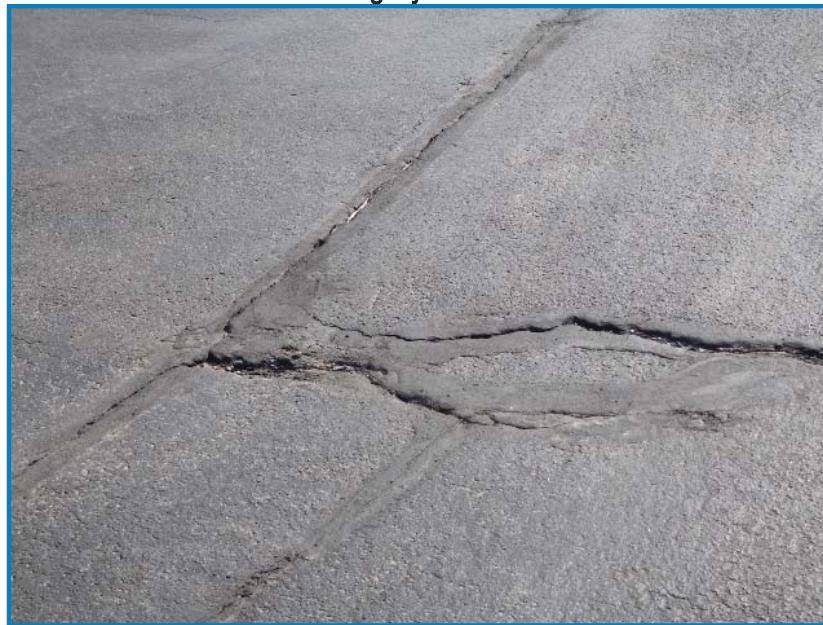
Typical asphalt cracking
